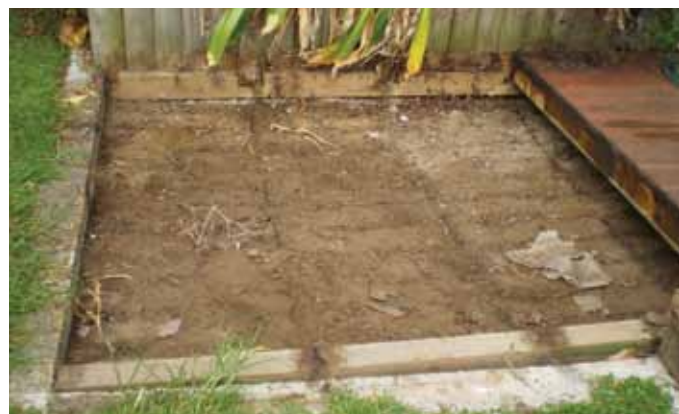
The septic tank in Paekakariki is covered in a sand layer, and located underneath a decked area.
