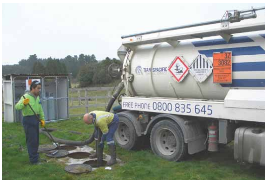
TK and Brad from Transpacific Technical Services extracting contents of the top tank into the 10,000 litre truck.
